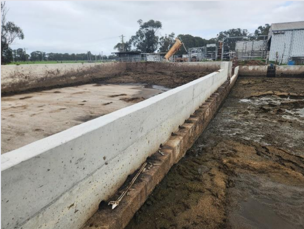
Concrete solids storage area (left) with bunded walls and drainage diverted back into the trafficable solids trap (right).
